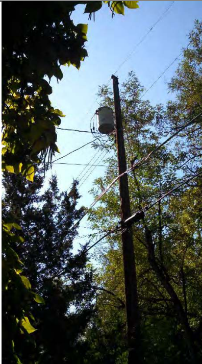
Photograph 19: Non-PCB labeled electrical transformer observed along the southeastern site boundary. View looking to the southeast. Staining was not observed on the transformer casing or on the ground beneath the transformer.
