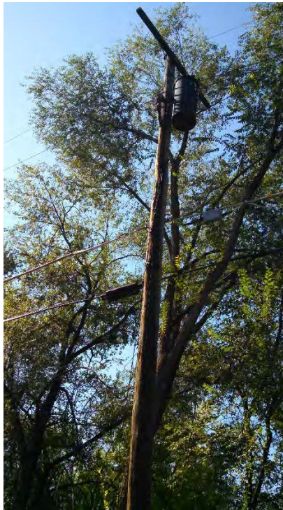
Photograph 20: Unlabeled electrical transformer observed near the north-center site area. View looking to the south. Staining was not observed on the transformer casing or on the ground beneath the transformer.
