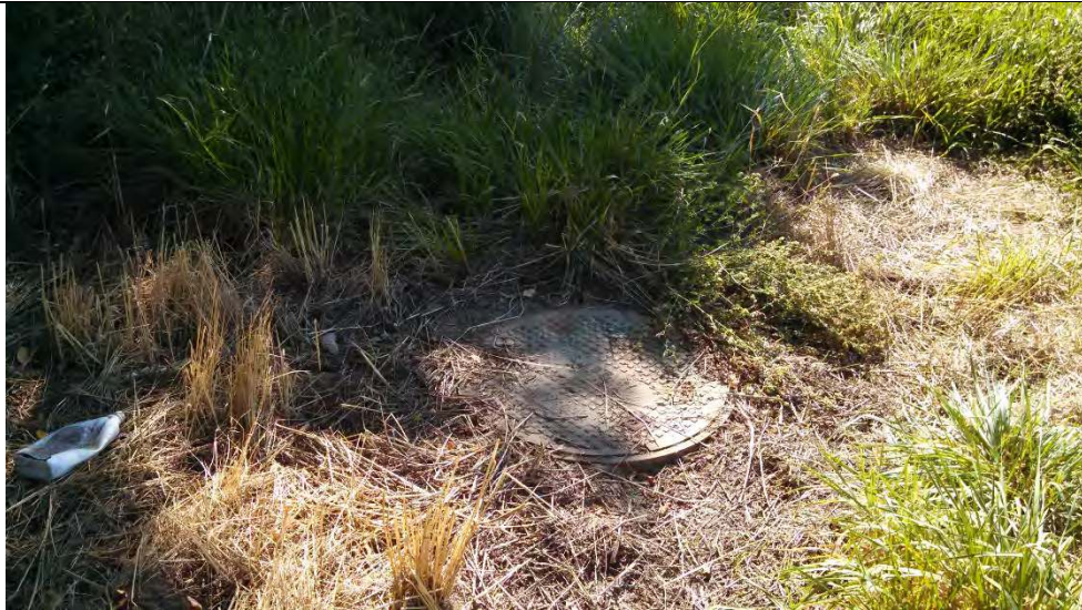
Photograph 30: Sanitary sewer manhole cover observed in the northwestern site area. City of Boise sewer line traverses the site from W. Moore Street southwest to N. Whitewater Park Blvd.
